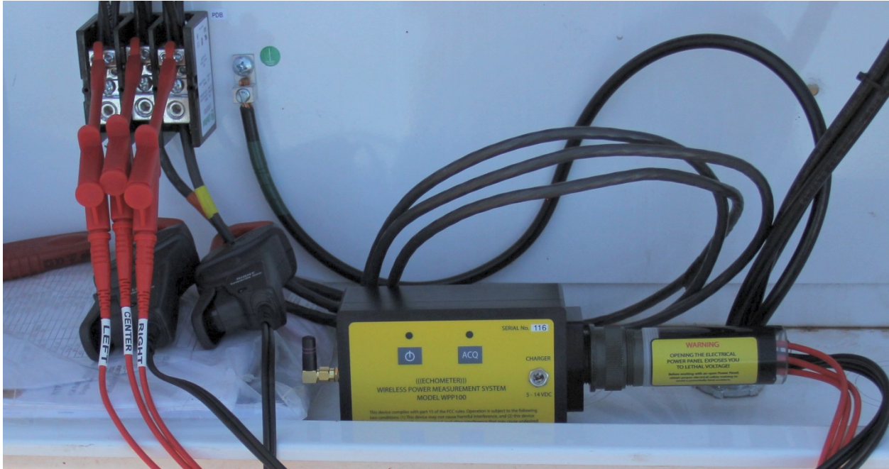
Figure 3 – Wireless Power Sensor connected to the wiring harness used to attach the current and voltage leads when an external connector is not permanently mounted outside the electrical switch box.
